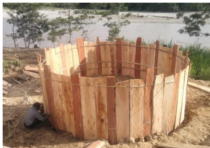
Figure 5. Securing wooden planks around the circular base of the Honai with rattan
