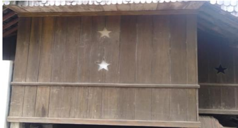
Figure 8. Darussajidin Mosque Air Ventilation
